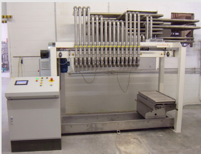
Gravimetric filling installation for 32 components by means of a moveable scale. All components connected by piping to fixed tanks and exchangeable IBC containers.
