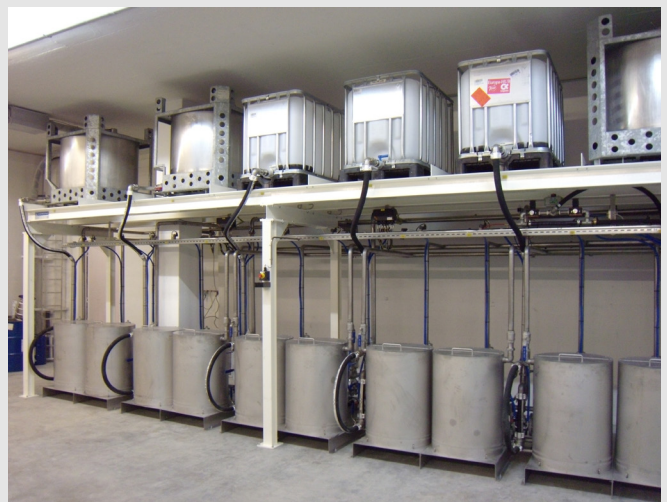
Example of a tank park with tanks and exchangeable IBC containers.
